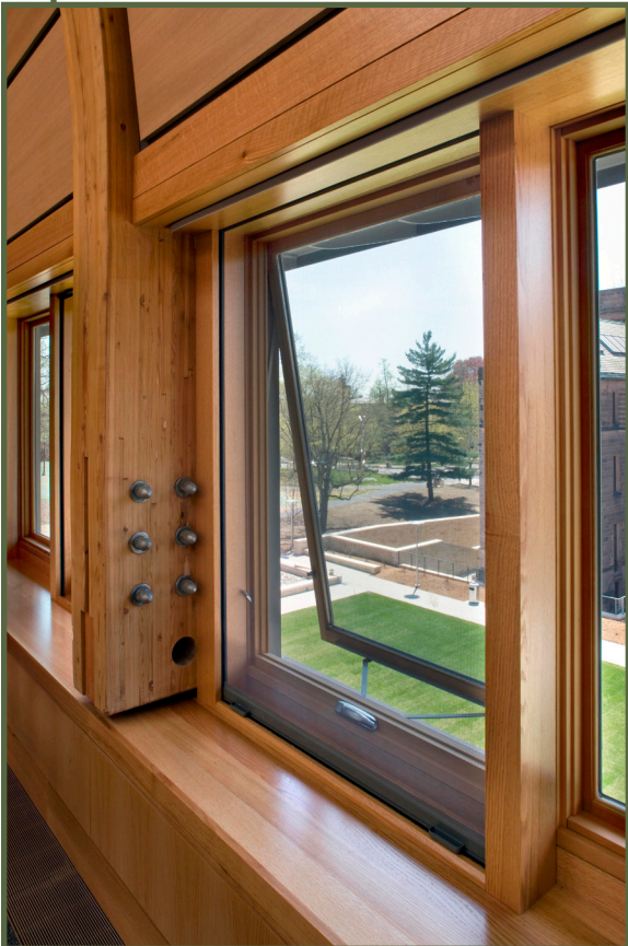
Below: Red oak was used for all the internal woodwork, with the exception of the glulam beams.
