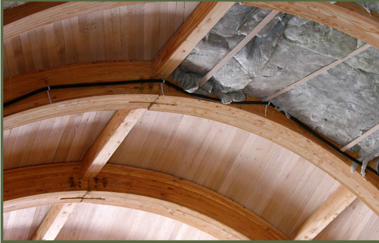
Two layers of North American ash connect 17 arches. One layer is fixed to the underside of the arch members, while the other is fixed to the upper face.
